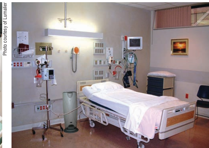
PHOTO B. UVGI recirculation unit on floor, alongside bed.
