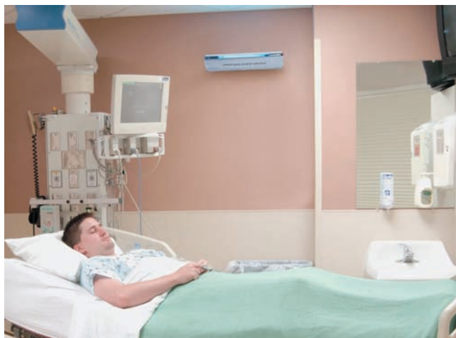
PHOTO A. Upper-air UVGI system installed in an ICU.
