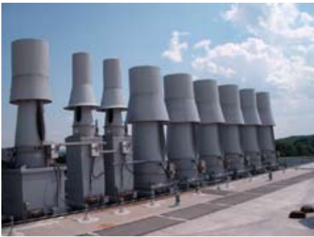
Figure 2 Low profile of Tri-Stack laboratory exhaust systems presents an unassuming roofline.
